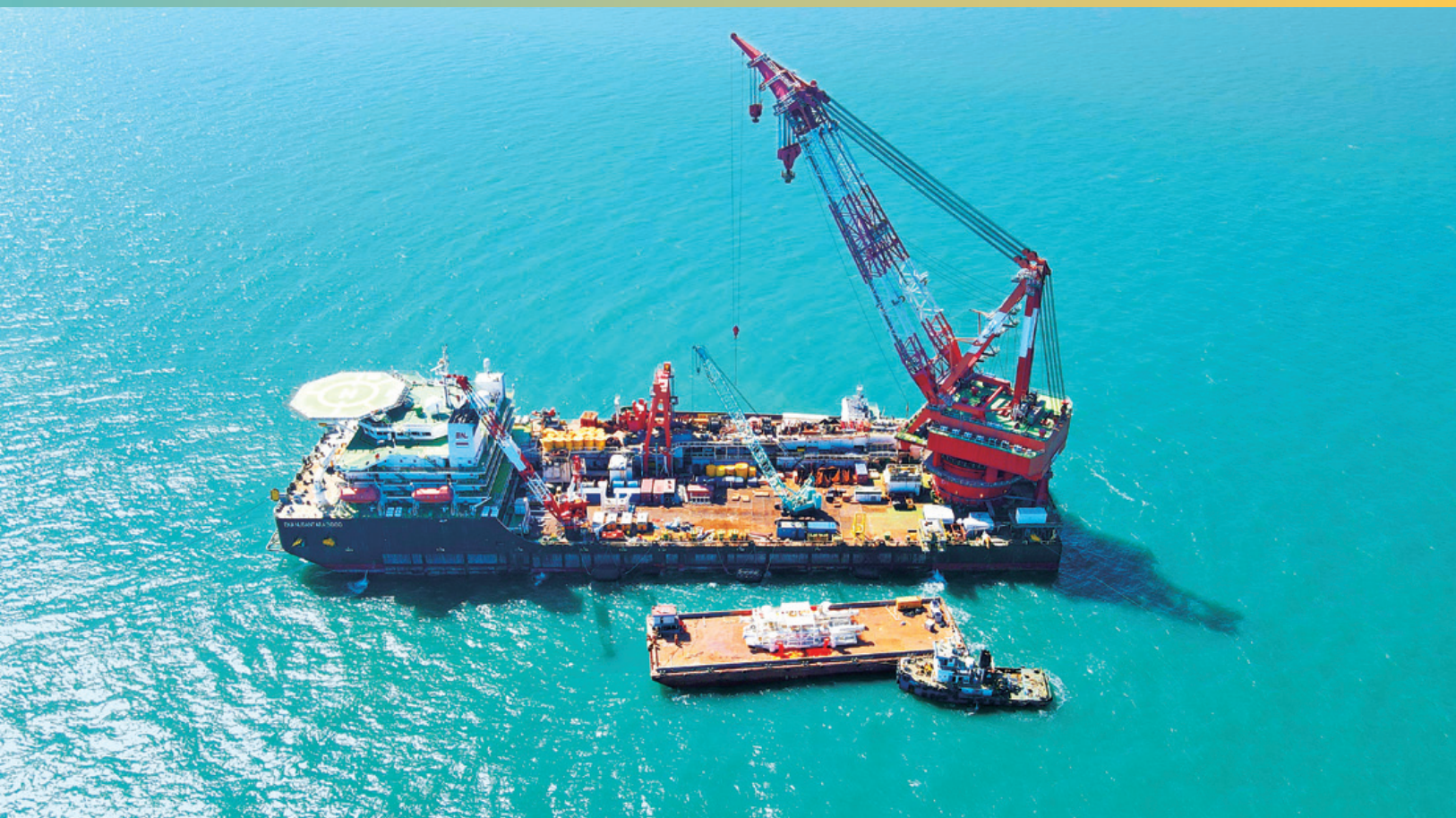
▲ Bangladesh Single Point Mooring (SPM) and Dual-Pipeline project, Bangladesh's first mega sea-land oil storage and transportation system built by CNPC
