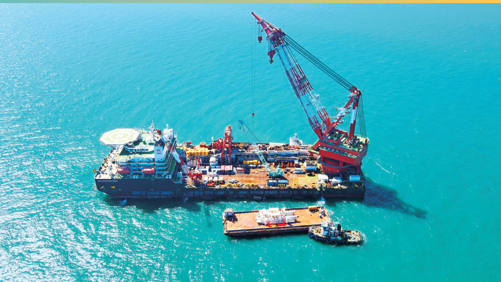
▲ Bangladesh Single Point Mooring (SPM) and Dual-Pipeline project, Bangladesh's first mega sea-land oil storage and transportation system built by CNPC
