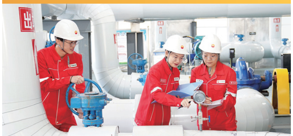
▲ Geothermal device check
