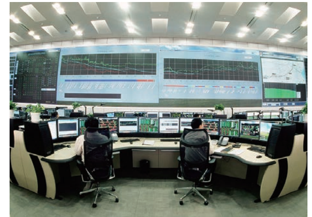
↑ Integrated controlled center
