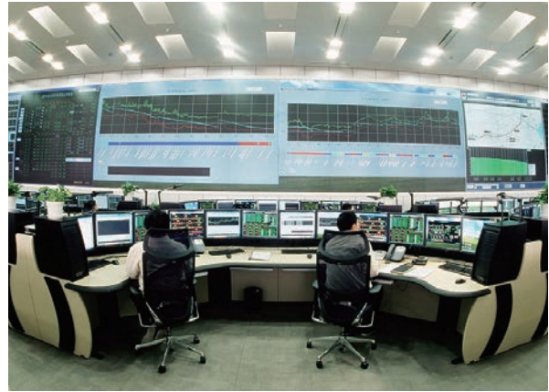
↑ Integrated controlled center
