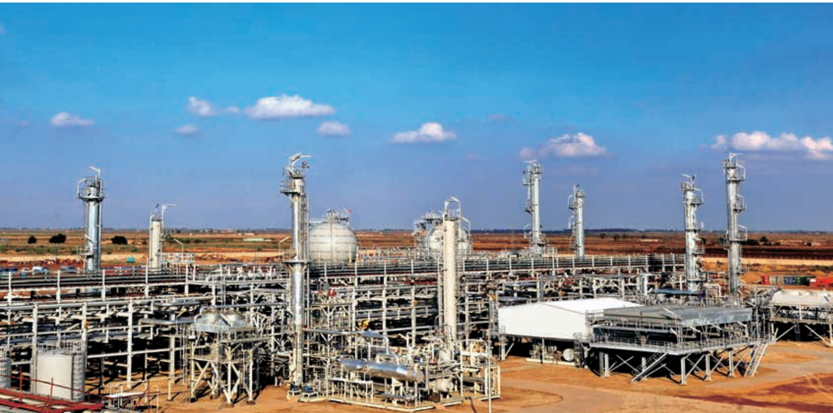
Al-Ahdab project is the first newly-built oilfield to become operational in Iraq in the past 20 years
