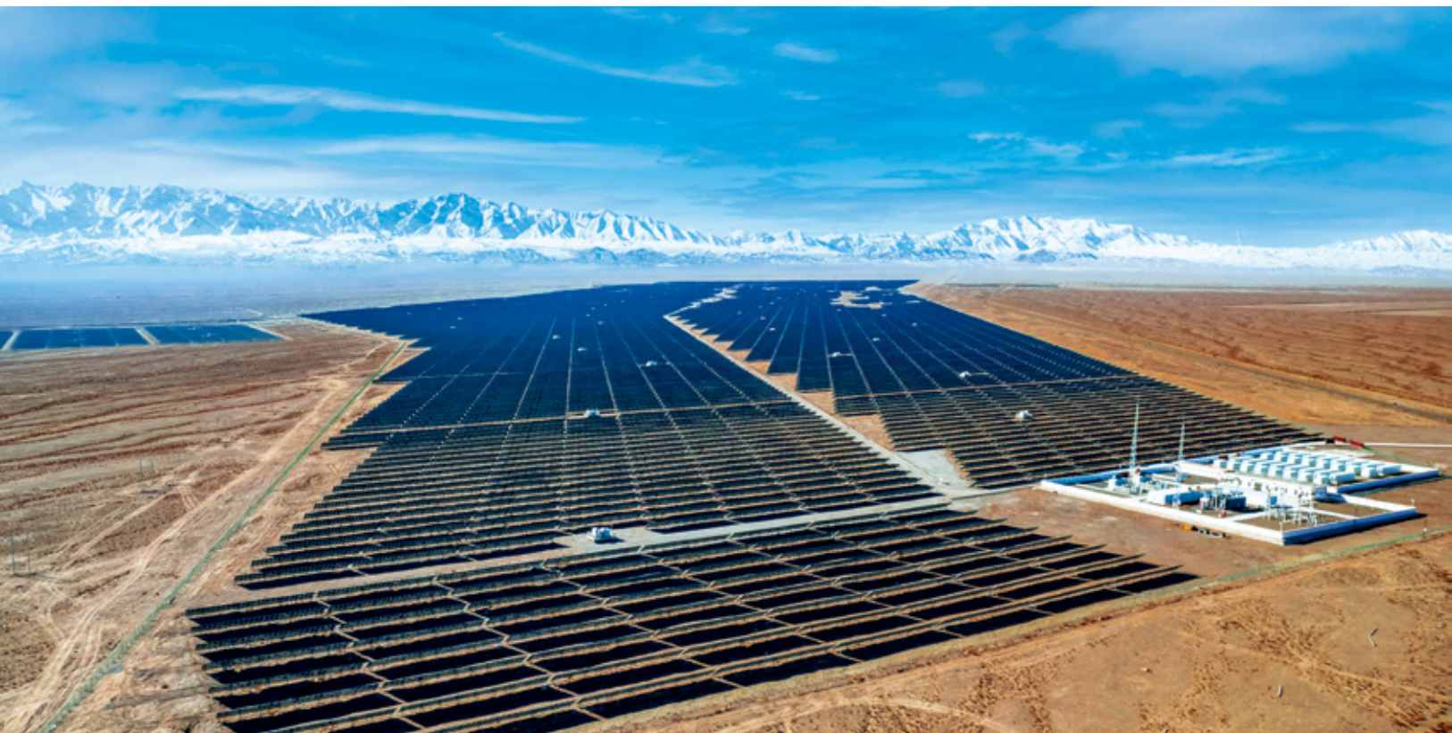
Yumen Oilfield's PV power project
