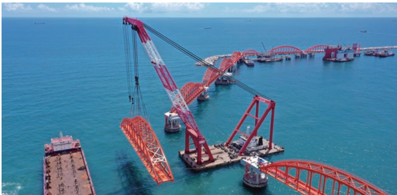
The crude oil terminal construction site of the refining-petrochemical integration project at Guangdong Petrochemical
