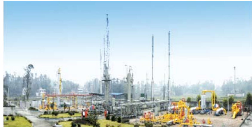
Datianchi dewatering station
