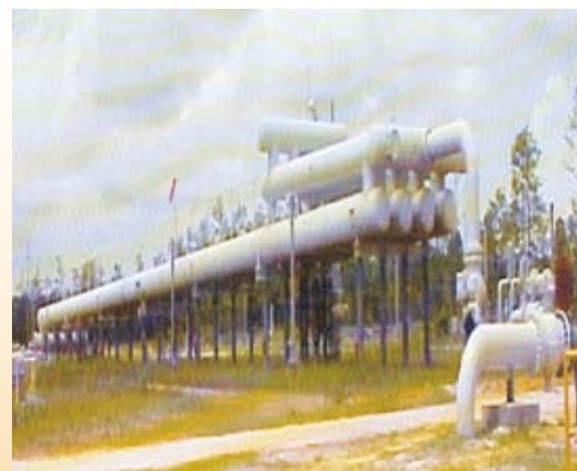
Liquid plug collector at the entrance of processing plant
