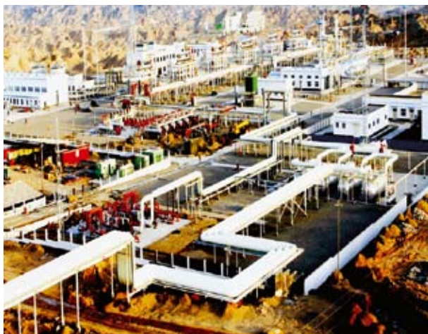
Central processing plant in Kela-2 gas field
