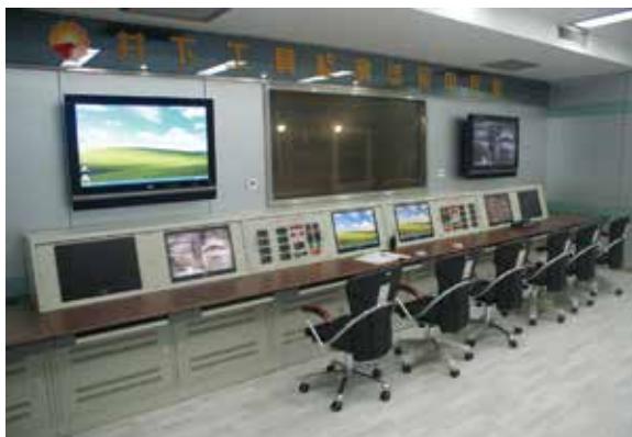
Remote control terminal of the system
