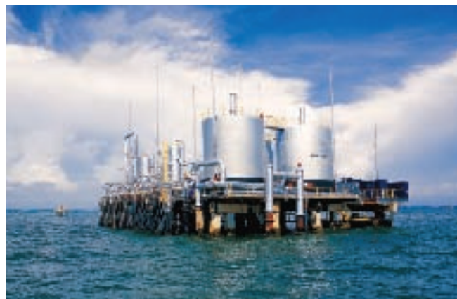
CNPC's transfer stations in the Maracaibo Lake in Venezuela
